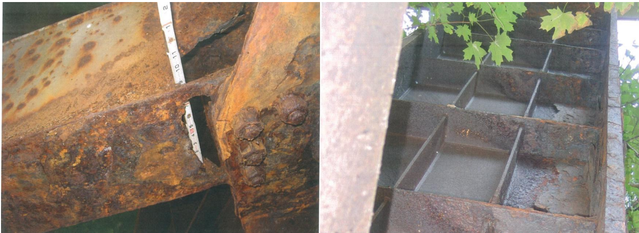
Figure 4. Section loss on lower bracing of northwest bridge leg (left image) and corrosion damage on southwest bridge leg below bracing (right image). (Source: September 2005 inspection report)
