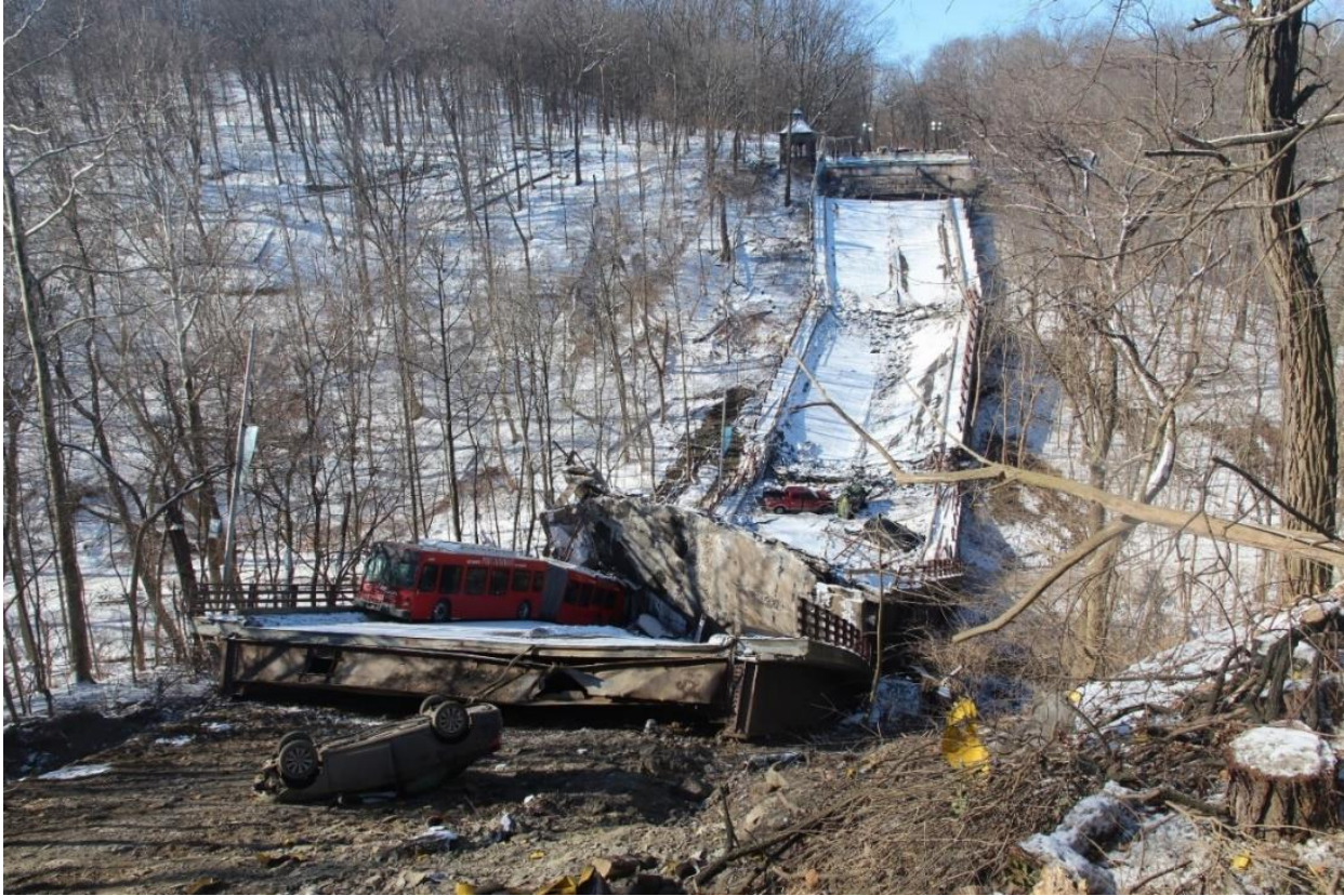
Figure 1. View of collapsed Fern Hollow Bridge from the east.
