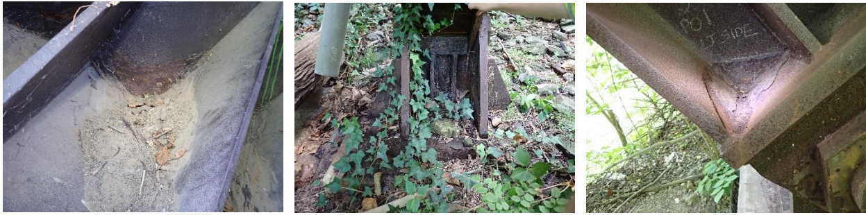
Figure 8. Photographs of built-up debris, lack of drainage, and associated corrosion on Fahy Bridge in Bethlehem, Pennsylvania (left); McCallum Street Bridge in Philadelphia, Pennsylvania (middle); and Shenango Road Bridge in Darlington, Pennsylvania (right).
