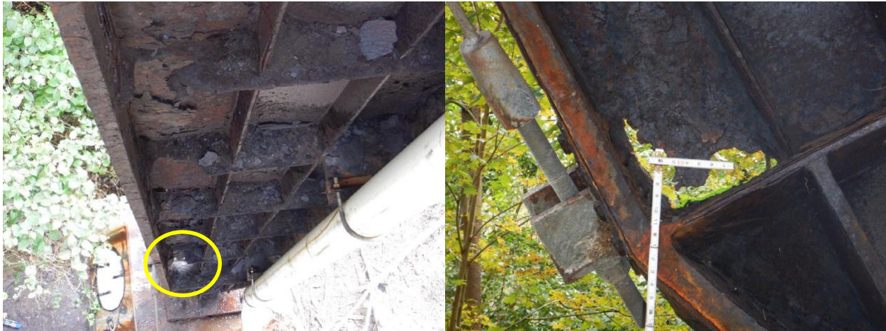
Figure 5. Corrosion damage including areas of 100% section loss on southwest bridge leg near connection to reinforced concrete thrust blocks (circled in yellow in photograph on left and shown in closer view in photograph on right). (Source: September 2021 inspection report)
