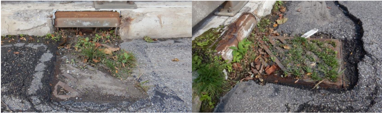
Figure 7. Blocked drains on Fern Hollow Bridge. (Source: September 2021 inspection report)
